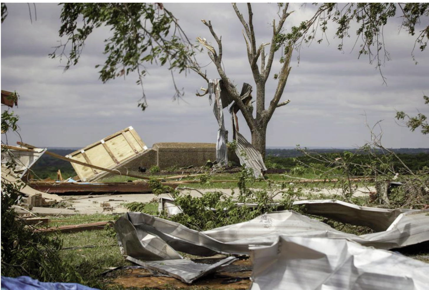
Metal parts of roof are tangled in a tree after a tornado near the storm shelter at the Barn on the Brazos wedding venue Tuesday, May 4, 2021, in Blum, Texas. Curtis Haley took shelter there as the storm hit Monday evening. (Yffy Yossifor/Star-Telegram via AP)
