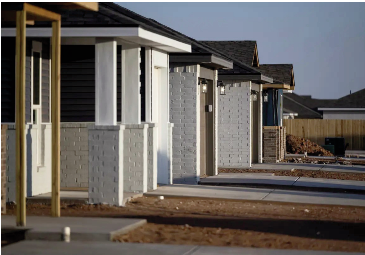
Homes under construction in a future neighborhood Wednesday, April. 26, 2023, near Wolfthorh in Lubbock County. Photo Credit: Justin Rex for The Texas Tribune
