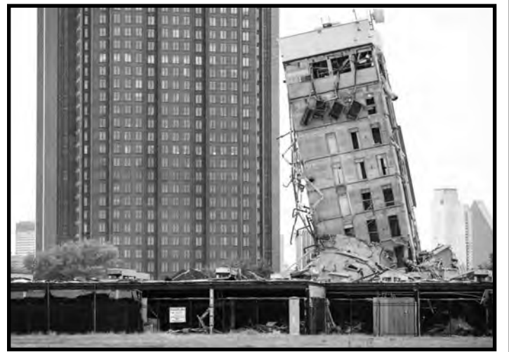
The former Affiliated Computer Services tower core shaft remains standing on Monday, Feb. 17, 2020 in Dallas. A demolition on Sunday morning left the single tower behind. (Juan Figueroa/The Dallas Morning News via AP)
